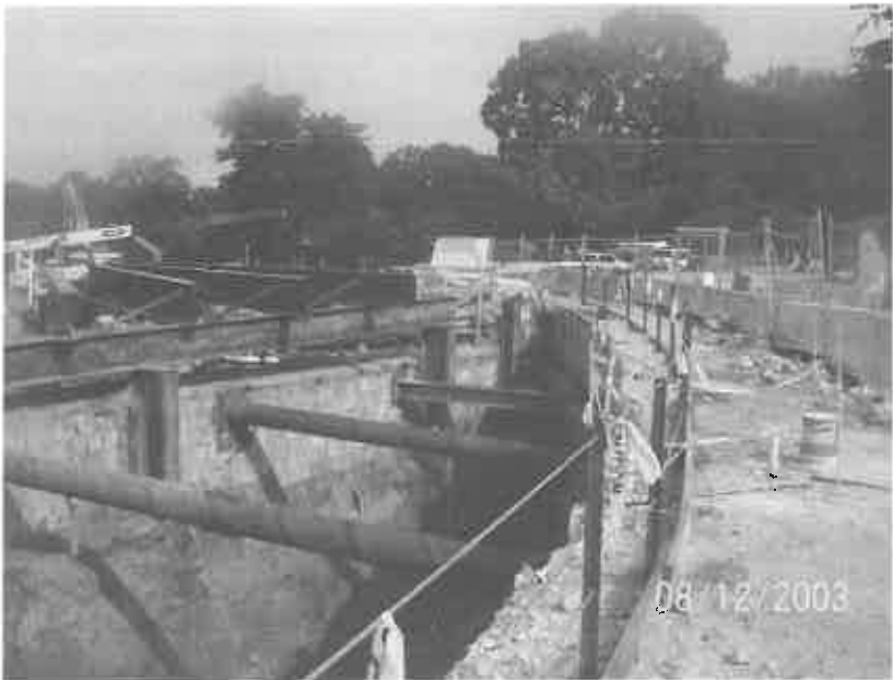
Figure 7 - Russell Tunnel Support System
