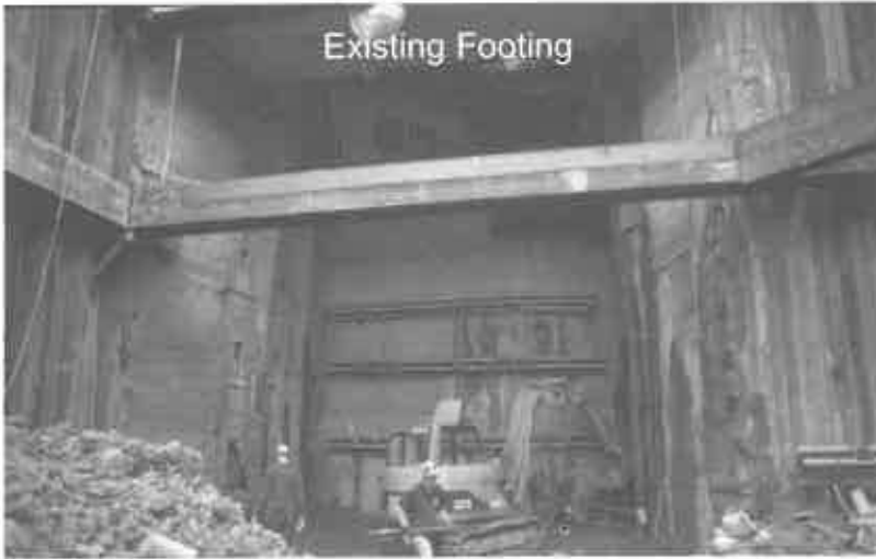
Figure 7: East Pavilion - Excavating to final tieback tier in new elevator & stairwell area.
