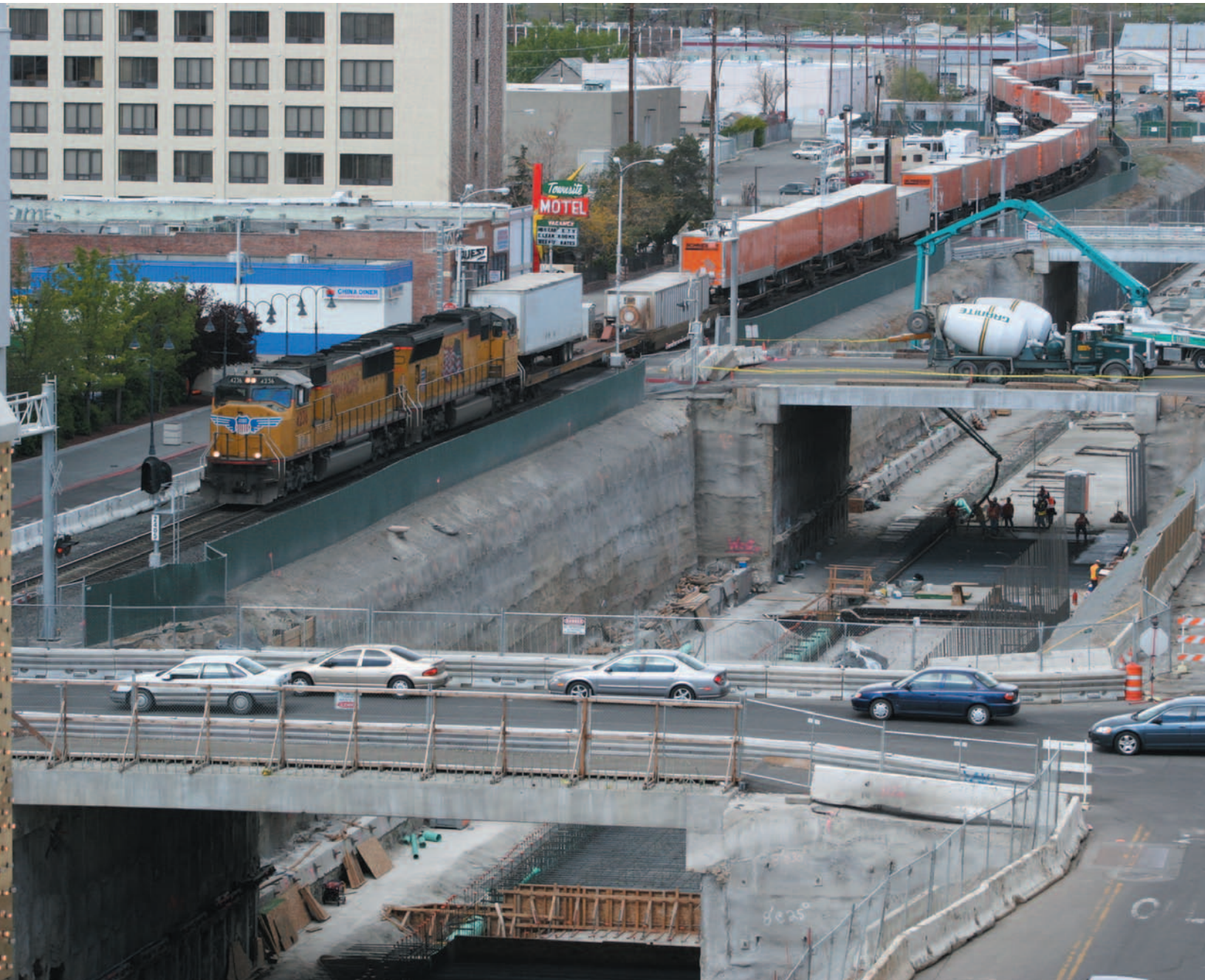
View of ReTRAC Trench spanned by temporary bridges, showing soil nail and shotcrete retaining wall subjected to Cooper E-80 train loading from shoofly
