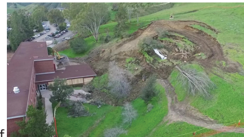
Landslide running into the Fremont Dorm
